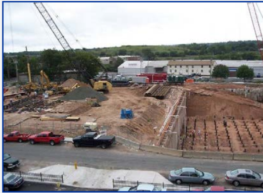
Underground Storage Tanks
