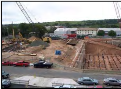
Underground Storage Tanks
