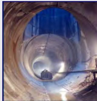
One Deep Conveyance Sewer
