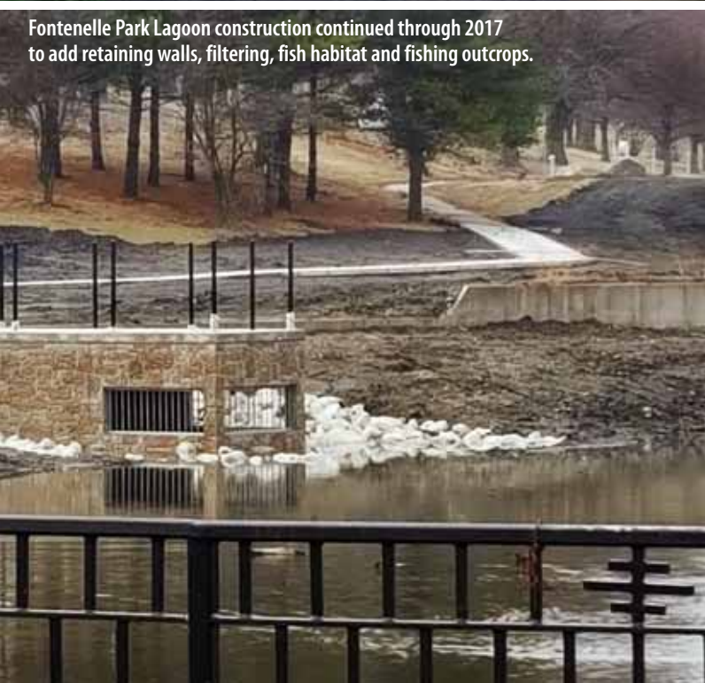
Initial grading to expand and deepen the Fontenelle Park Lagoon began in 2017.
