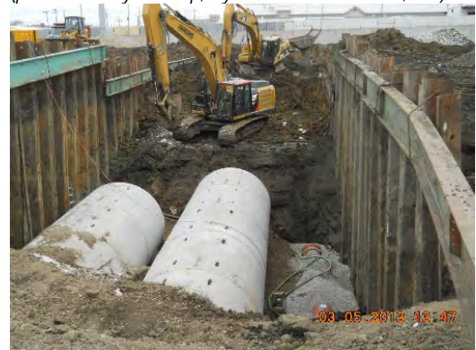
FIGURE 2-9 Pipe Installation during the Nicholas Street Phase 1 Project (photo courtesy of Lamp, Ryneerson & Associates, Inc.)
