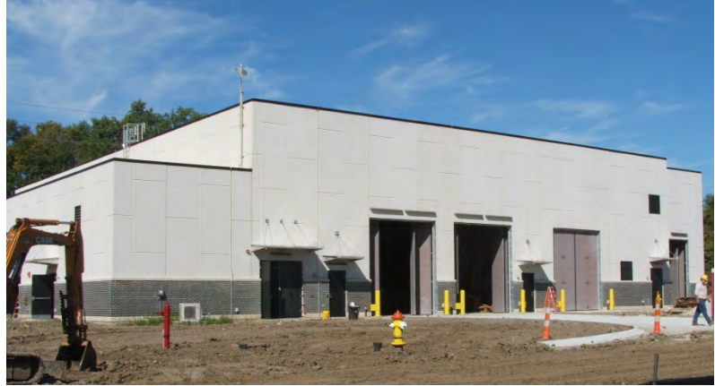
FIGURE 2-3 Leavenworth Lift Station (photo courtesy of HDR)
