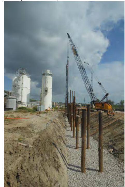
FIGURE 2-5 Construction of Schedule B1 at the MRWWTP (photo courtesy of CH2M HILL)
