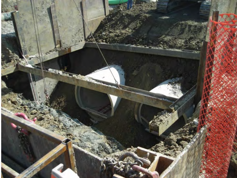
FIGURE 2-10 Construction of the Nicholas and Webster Phase 1 Project (photo courtesy of City of Omaha)
