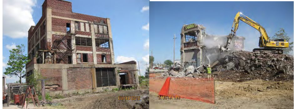
FIGURE 2-8 Economy Products Building Before and During Demolition (photos courtesy of Lamp, Ryneerson & Associates, Inc.)
